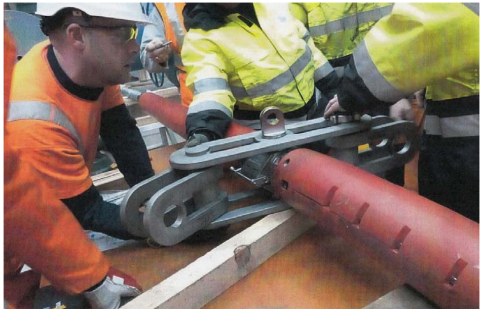
Installation of the PMI Dyna-Hanger cable hanger and Dyna-BSR bending strain relief systems.
