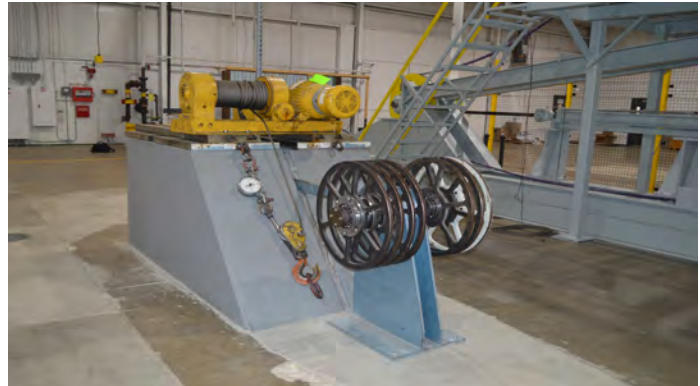
Long span tension setup
